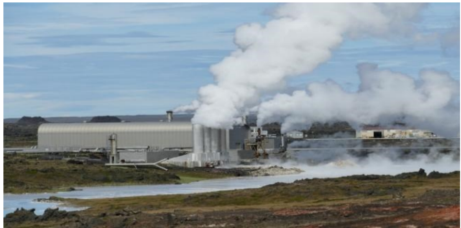
Figure 25. Geothermal power plant.
