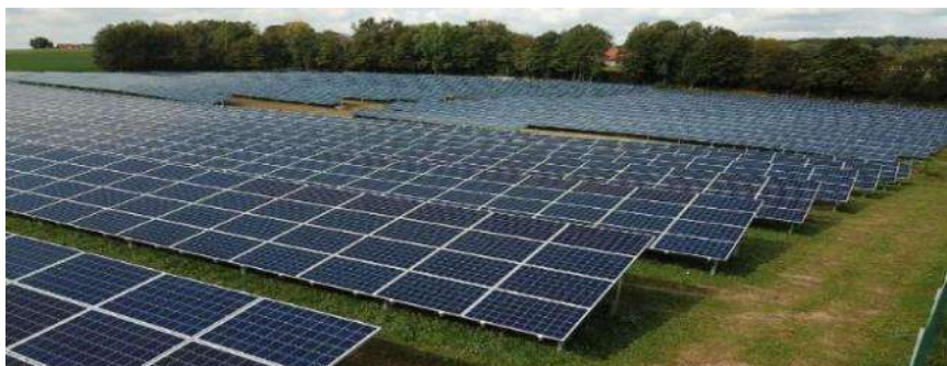
Figure 17. Solar PV park.
