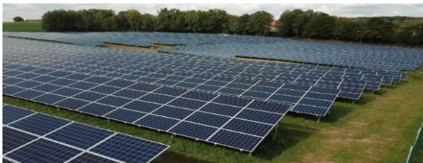
Figure 17. Solar PV park.
